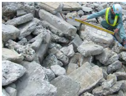
(Quake concrete Wreckage)
