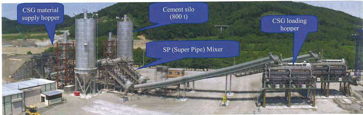
Photo-17 CSG Production Equipment (Tobetsu Dam)
