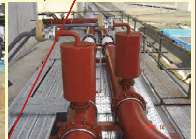
Conveyance unit - Sediment discharge pipeline & pressure regulator
