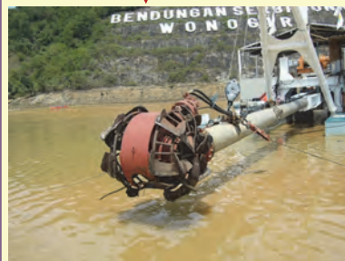
Siphon intake unit - Siphon Barge
