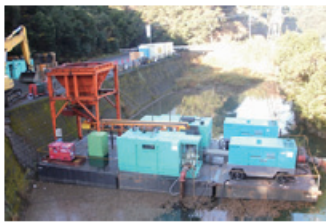
Feeding system (Hopper station)
