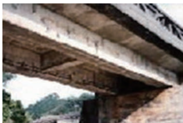
Bridge (chloride induced deterioration)
