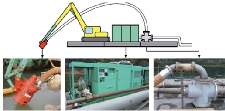
Screw crusher High pressured pump Special ejector
