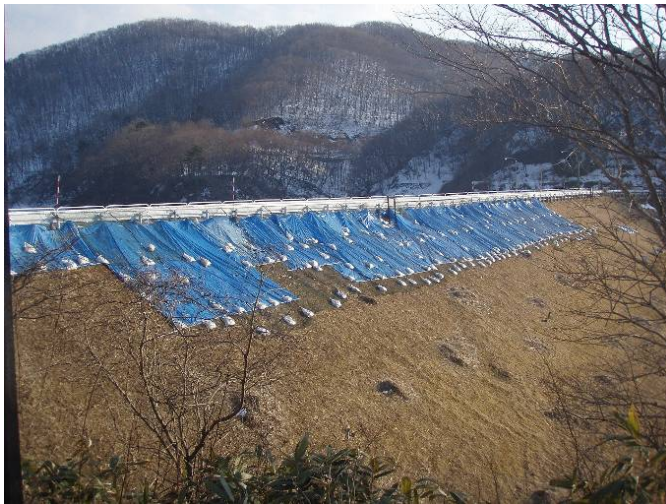
Figure 10. Hatoriko downstream slope
