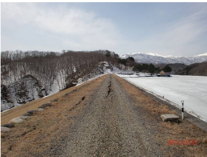
Figure 11. Nishigo Dam; cracking on the crest
