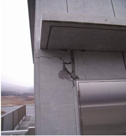
Figure 5. Cracking at gate house
