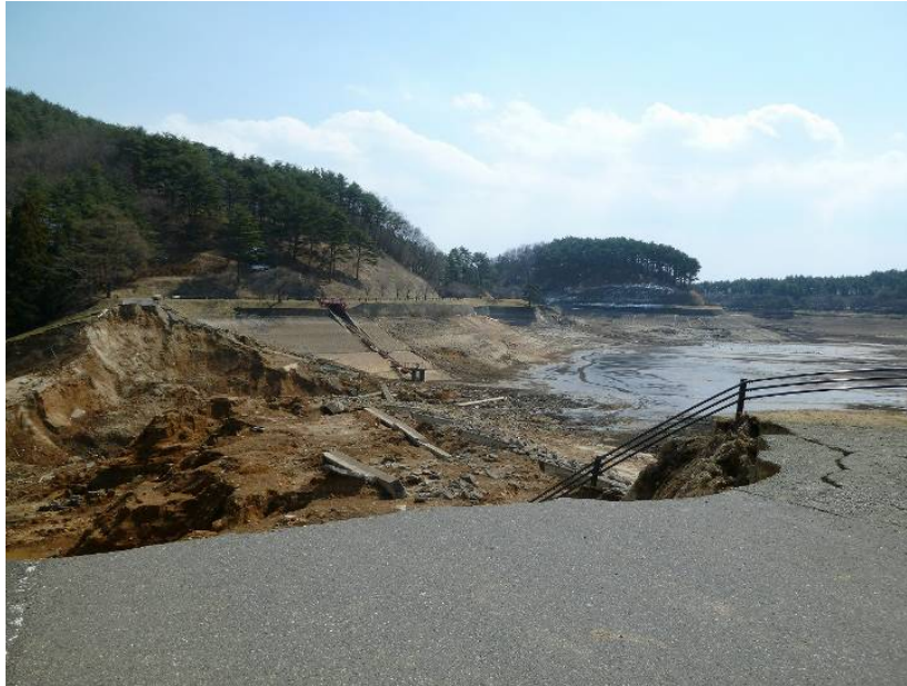
Figure 14. View from left abutment toward the breached portion
