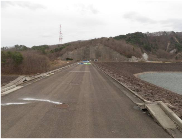
Figure 6. Bump on the crest of Nanakita Dam
