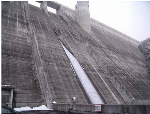
Figure 4. Takou Dam after the quake
